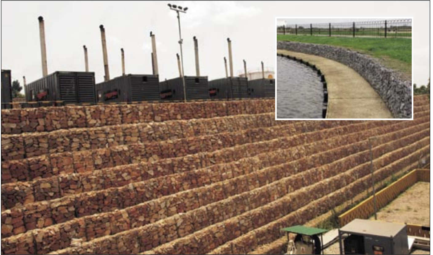
▲ 10m high mass gravity woven wire gabion wall designed and constructed in Kampala, Uganda.
