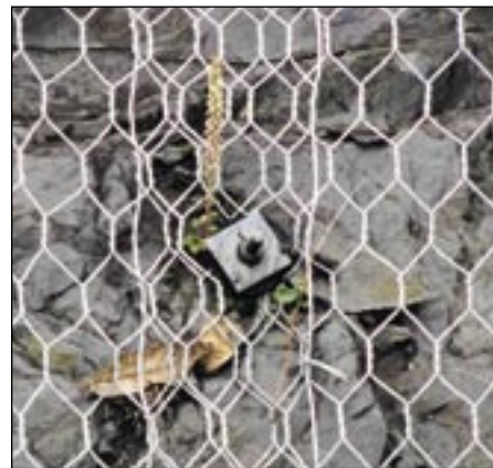
◀ A typical photograph illustrating rock fall protection netting draped and bolted to a cliff face to prevent debris from falling to the road below. ▼
